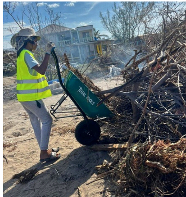
Debris Removal, Treasure Beach
